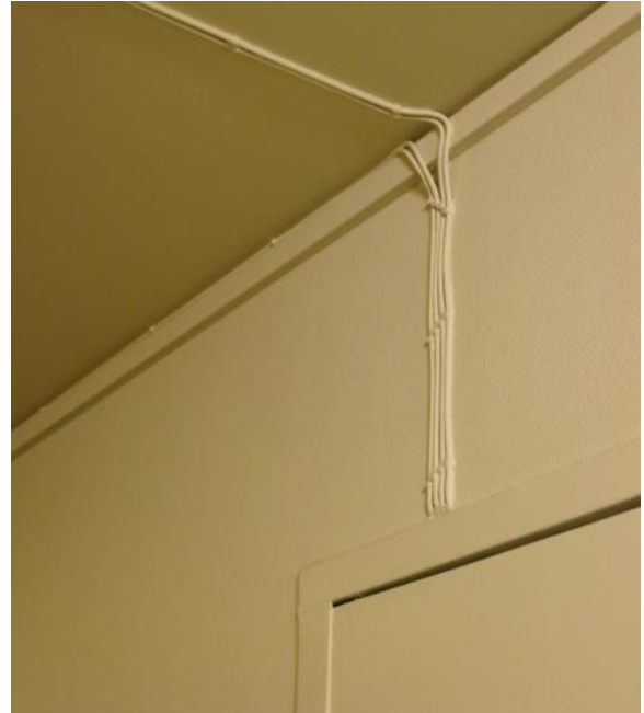
Electrical lines are replaced on all levels, more or less great need. Carried out by electrical contractor.
