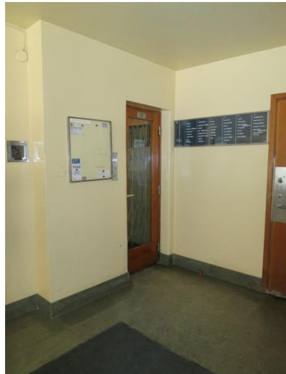
The notice board needs to be aligned and adjusted in height like the nameplate, for example. The bulletin board is not original as the nameplate is.
