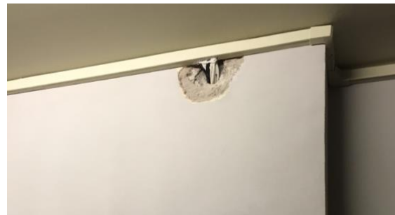
Vertical electricity- and fiber cables run in the elevator shaft and the new electrical duct at the ceiling has been drilled out. Sometimes the wall broke a little. Due to the very hard concrete, new installations could not be built into the walls.
