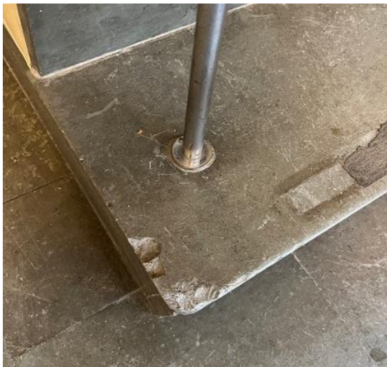
Damage to the limestone in the exposed stair corner
