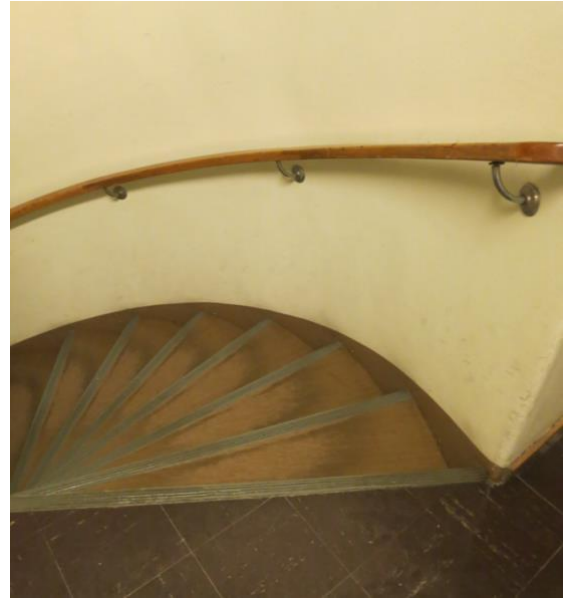
Worn stairs with painted plinth against the wall, probably from the 1970s.
