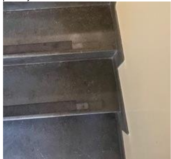
Worn out slip tape and traces of old tape.
