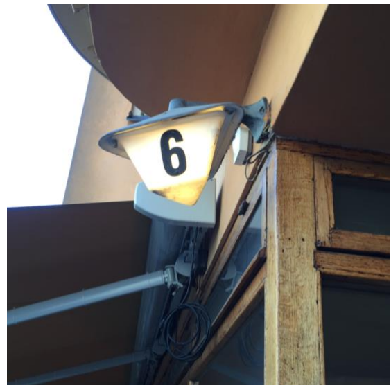
The outdoor fixture replaced with a standard fixture from the 1960s-70s, a little tufted.
