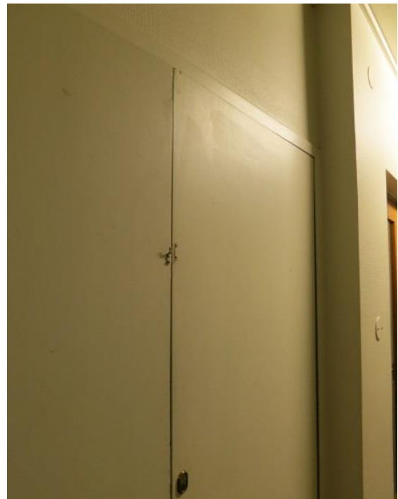
Existing fittings for hatches are supplemented and fixed by carpenters before painting.
