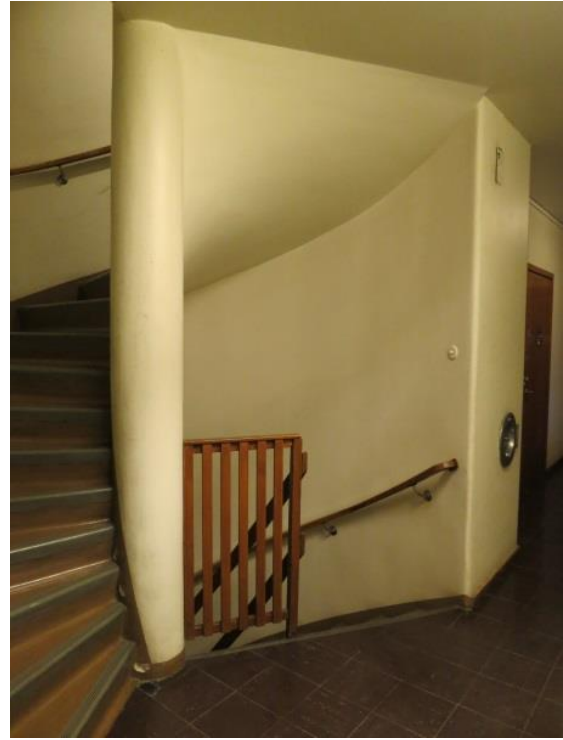
Take a stand on the existing railing to the basement. Compare with the stair railing to the entrance floor, below.
