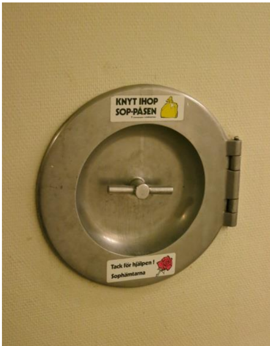
New text about GARBAGE SHAFT and former LAUNDRY SHAFT is stenciled over the respective hatch.
