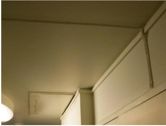
Electrical cords for fixtures are unfortunately routed across the corridor. The eaves against the ceiling contain, among other things, data and telephone lines.
